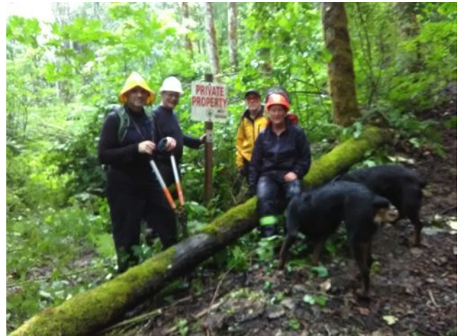
Crew work on the Tolmie side of the trail. Photo by Jim A
