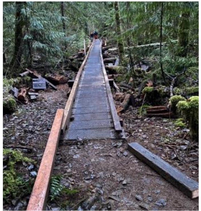
The finished 100 foot long boardwalk/bridge with the curbs and expanded metal mesh.
