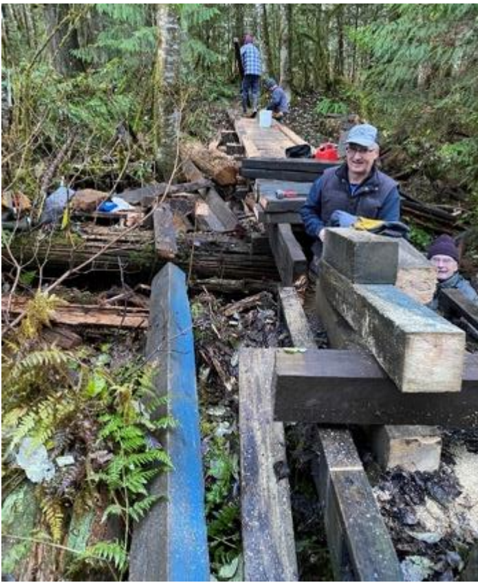
As the next section was constructed on December 12, the decking was cut and secured to the stringers, Tim added final blocking to secure the stringers and Don checked out the depth to the bottom of gully. Brand and Lorenz worked on the new curbs.
