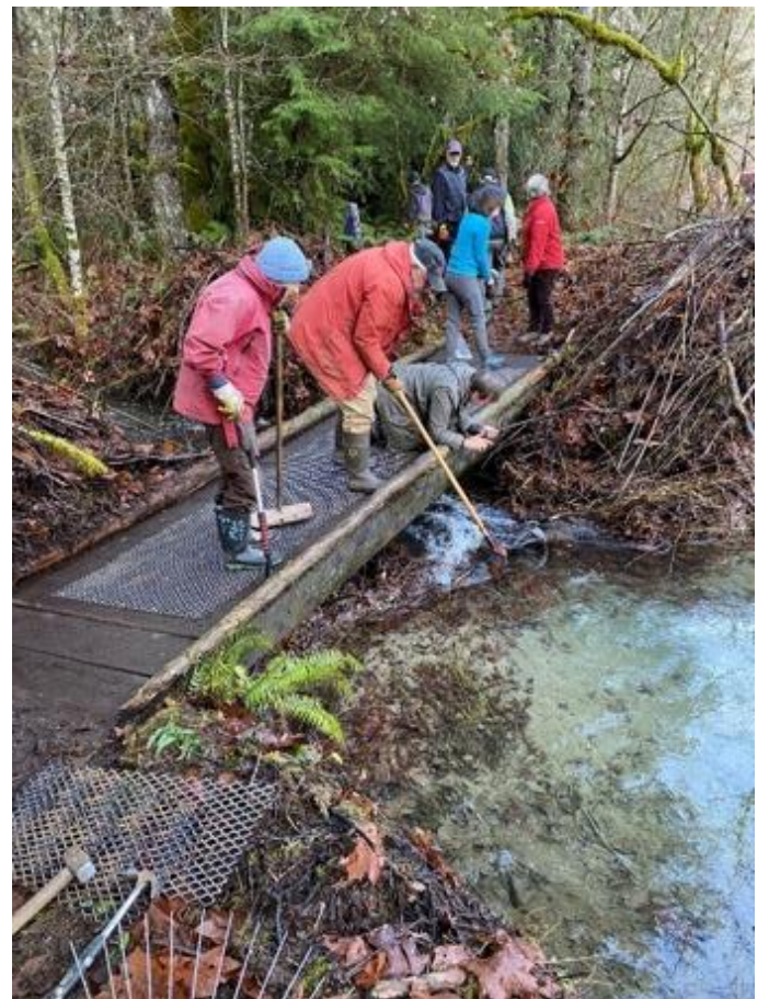
On December 15 the crew returned to add the expanded metal mesh 5 bridges in the Thurston Meadows section of the Trail and to the last section of the boardwalk east of Riverside.
