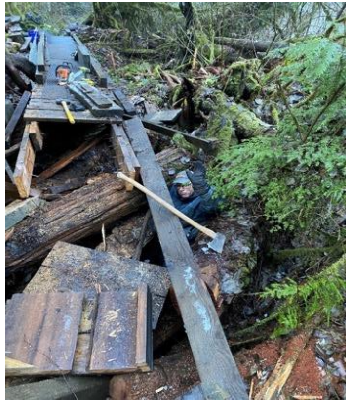
On 12 December we returned to complete the replacement of the last section on the boardwalk/bridge. The depth to the ground below the deck was about 8 feet and Jim S slipped down to check it out.
