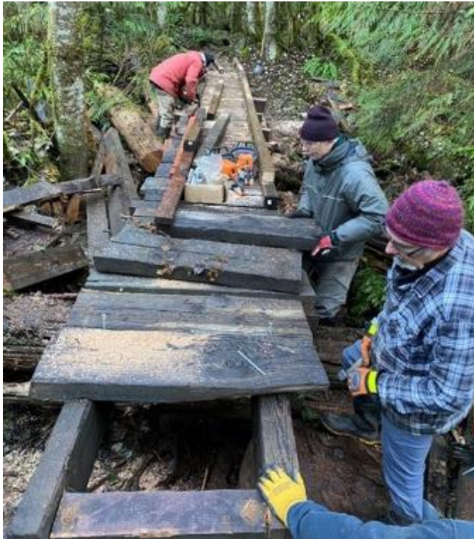
Next Don and Lorenz secured the decking to the stringers and Heinz and Brad secure the curbs along the completed deck.
