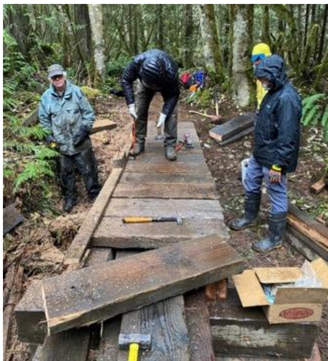
Patrick, Lorenz, Jim S, Gary added the curbs and trimmed the edge of the decking on the first section.
