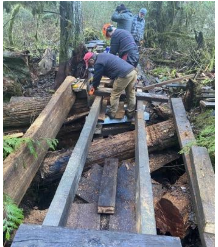
The process was repeated by removing the deteriorated deck and constructing new timber piers; the old cedar deadfall made the task of aligning the piers and the stringers
