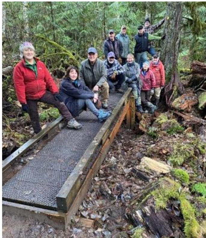
The Happy crew at the Riverside east board/walk bridge. Completing a major task brings a pride of the accomplishment to the team.
