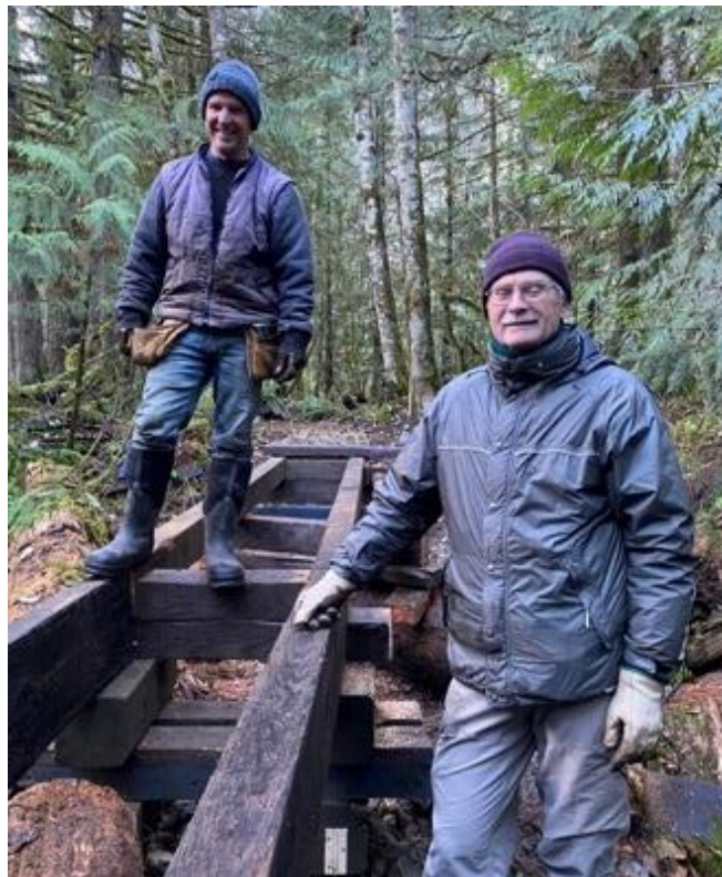
November 23 the crew replaced another section of the bridge. New piers were constructed using the 6"x6" timbers and the large stringers. Brad and Don work on connecting the stringers.
