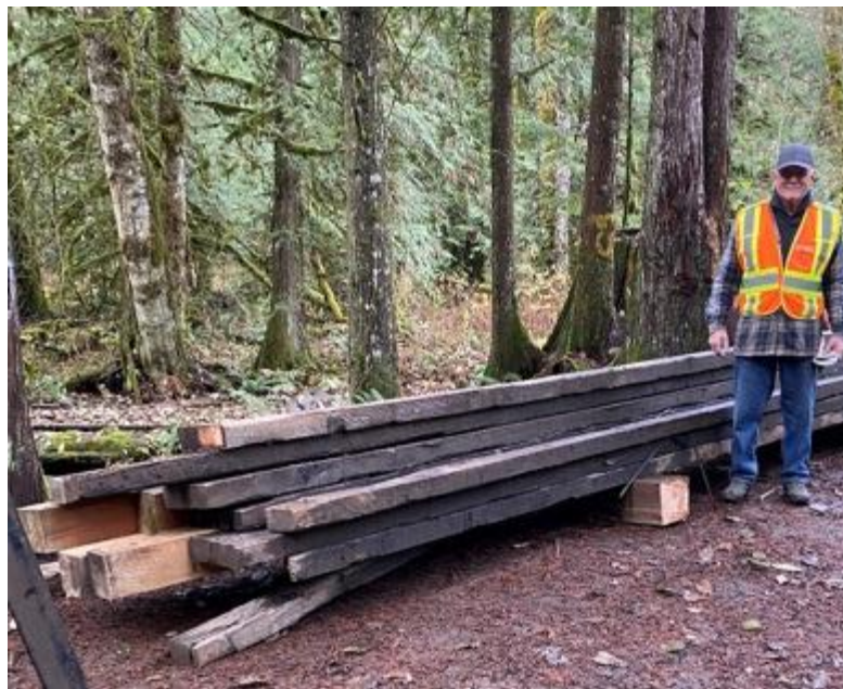
On November 20 additional material was brought in from Hunter Creek for the decking and stringers. The material was stockpiled at the trailhead campsite. Fortunately, only a few pieces of 6"x6" timbers were burned by campers.
