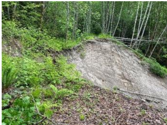
A major slide destroyed the rail bed near Carolin Road.
