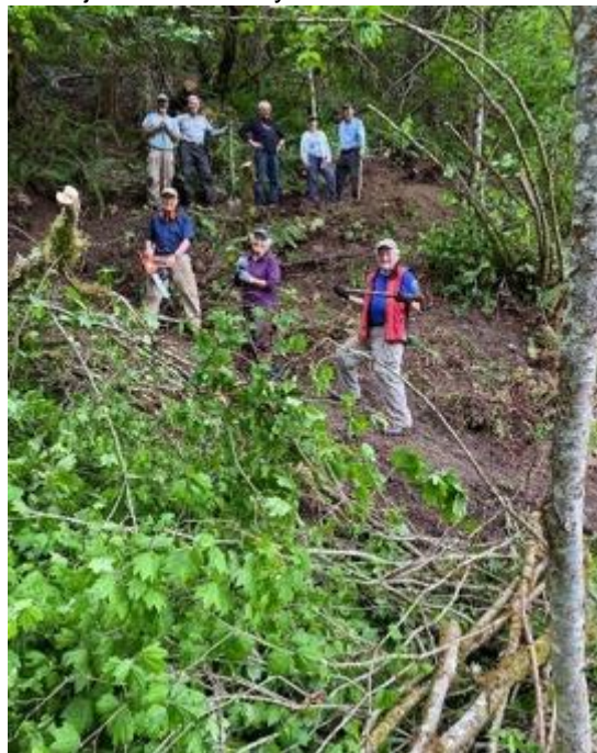
The eager crew Heinz, Em, Don, Rob, Serge, Leon, Deborah, Janet, Ray, Jim constructed a bypass trail for safe passage above the slide.
