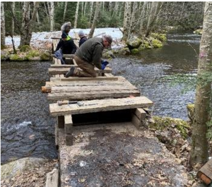
The railings were added using salvaged material Jim Shirk obtained plus pressure treated material COC previously purchased.
